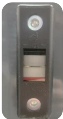
Sight glass for checking hydraulic oil level in tank
