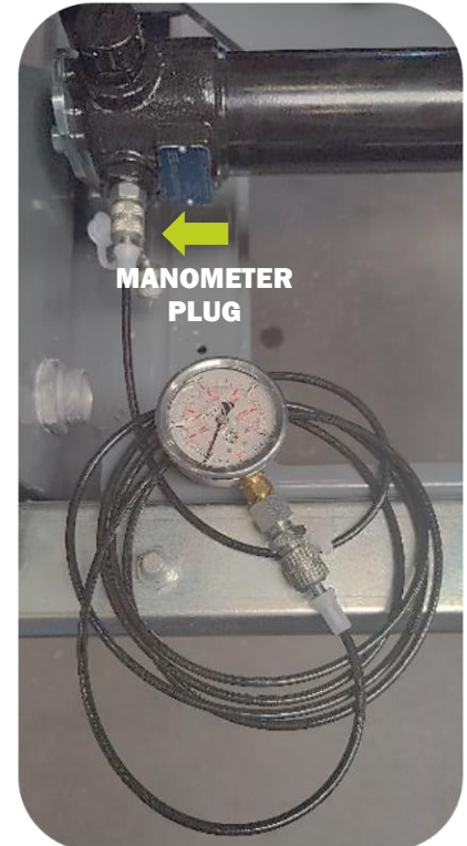
Connection of manometer at the outlet on the high-pressure filter
